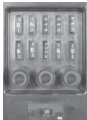
Figure 9 - Main Disconnect Switch
